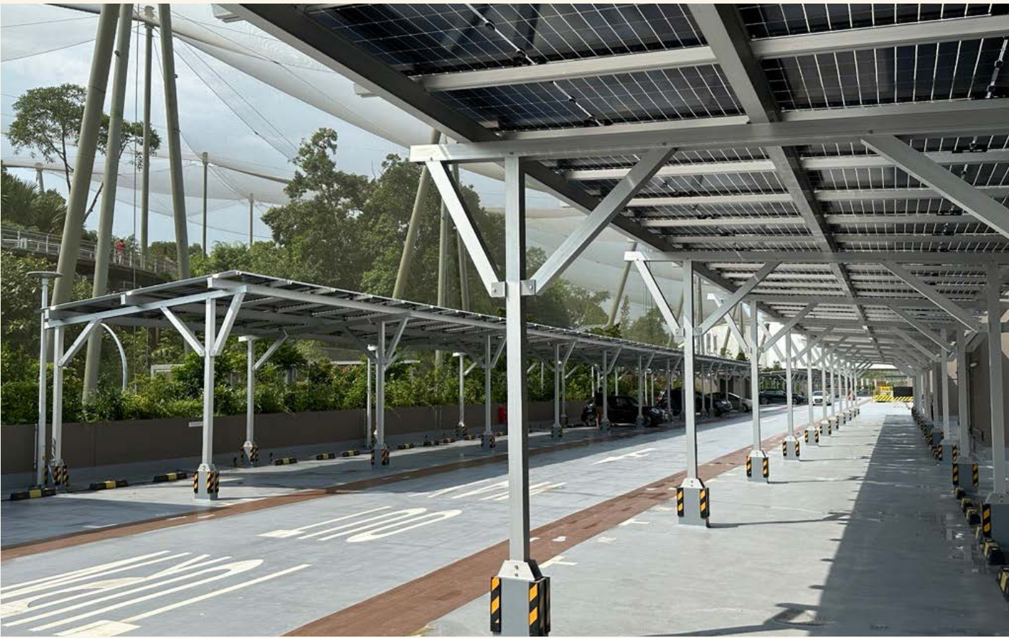
Solar panels in our carparks.
